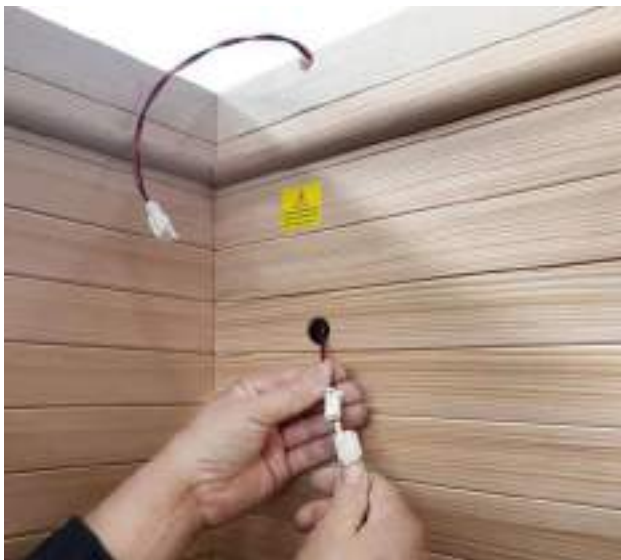
(9) Connect sauna light cable as above.
